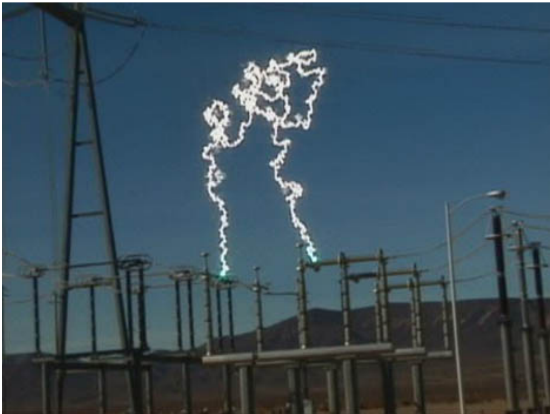
500kv Electric Arc - Vacuum Switch Failure
