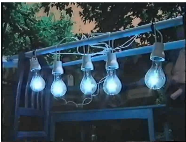
Figure 10. Generation of 5 kW of electricity in autonomous mode with the starter (battery) disconnected
