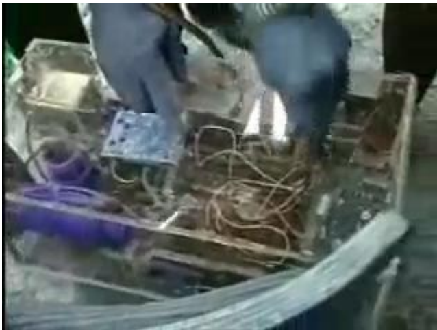
Fig. 15: Generator, top view
