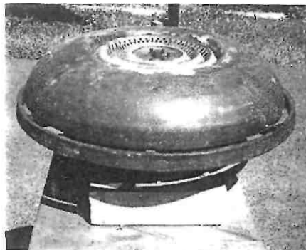
(c) Inner distributor cone removed to expose central portion of upper meander-plate.
